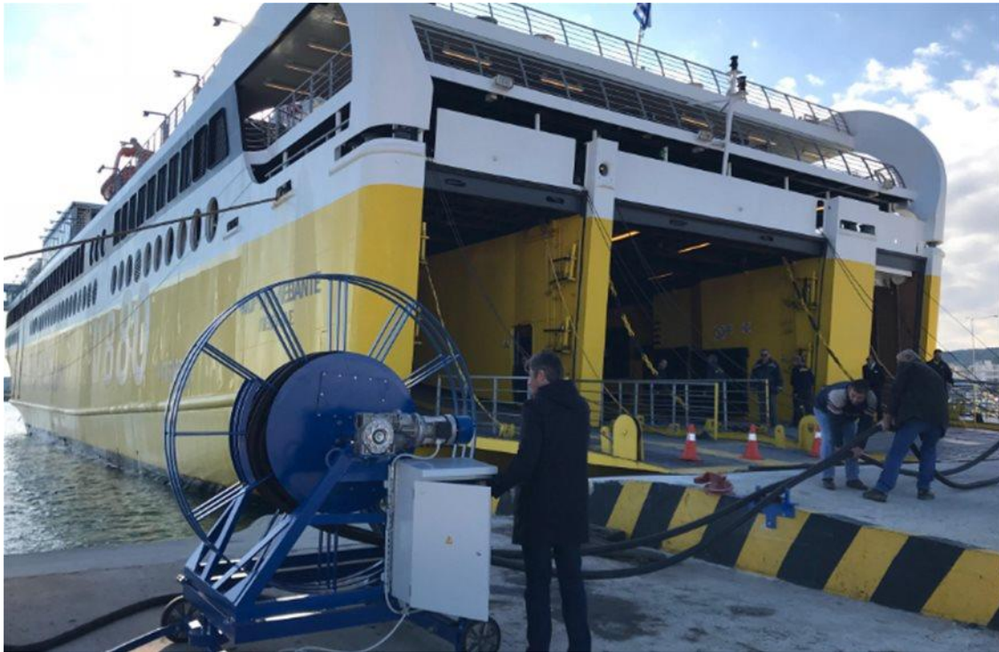
(Photo 2: Plug in of the passenger ro-ro ferry FIOR DI LEVANTE, with the first pilot installation for shore based electrification, port of Killini, 20/12/2018)
